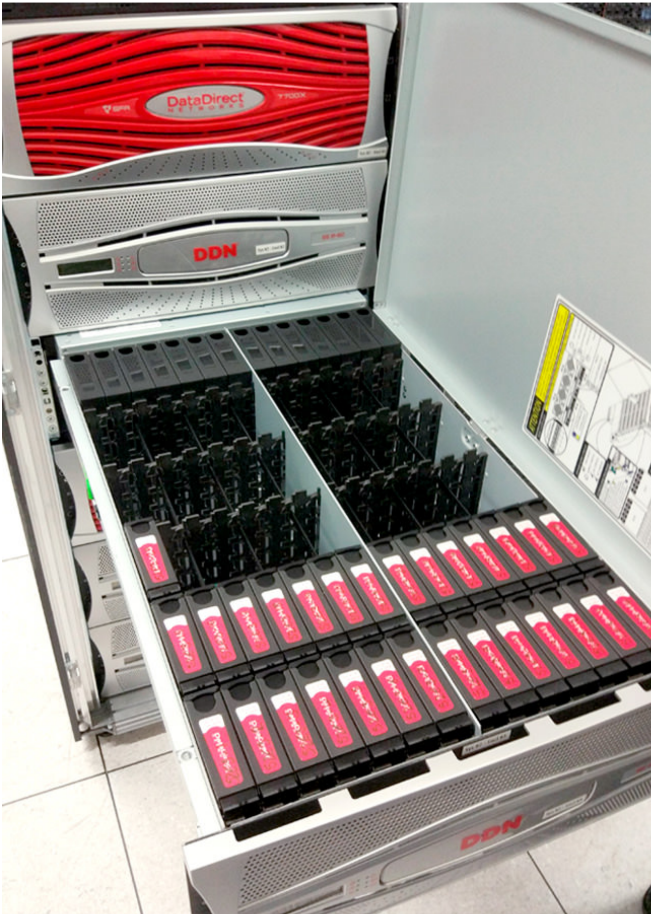
Barcelona Supercomputing Center
